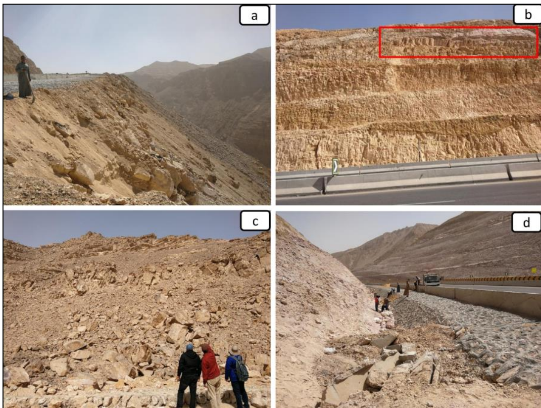
Fig. 15 Site photographs showing (a) the rock fragments and dump materials at the upper part of slope (seed area), (b) the hanging rock blocks in the slope face (propagation area) at the upper part (the red rectangle), (c) The dominant block size which ranges between 0.5 \text{ m}^3 to 3 \text{ m}^3 and (d) the constructed side ditch at the slope toe with width of 2.5 m
